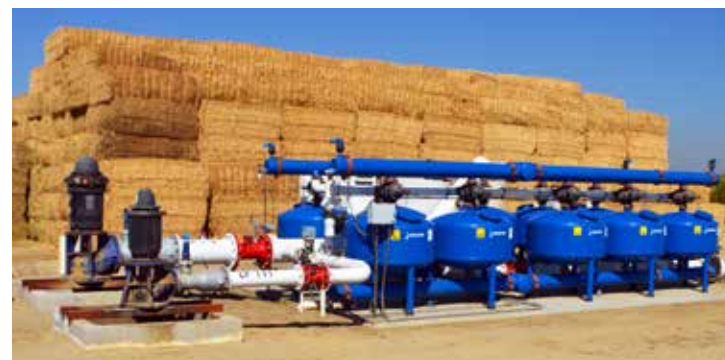
SDI-E Filter Station
