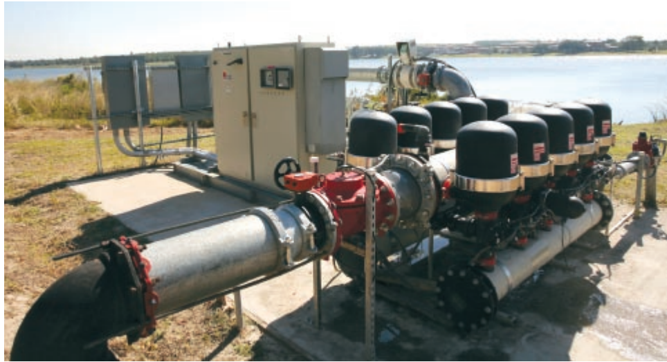
Source water from Lake Siena is pumped through Bella Collina's filtration system, Netafim's Galaxy Disc Filter, before being distributed to the irrigation pipes.
