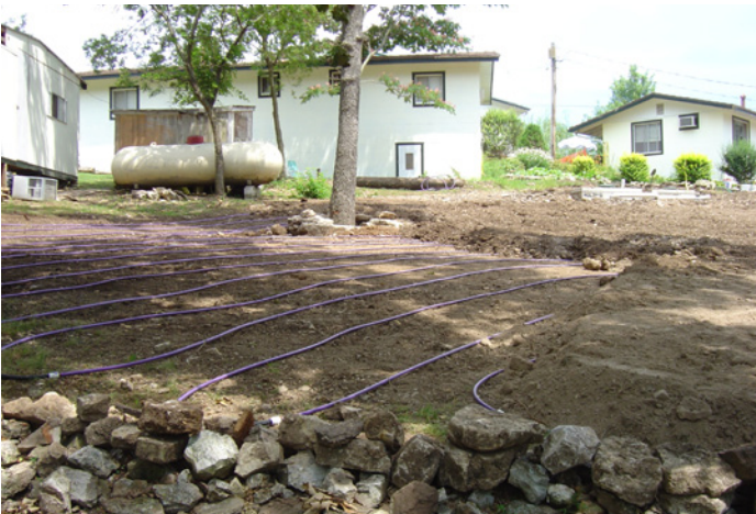
As shown above, when laying the dripperline on a slope, it is recommended that the dripperline be laid perpendicular to slope.
