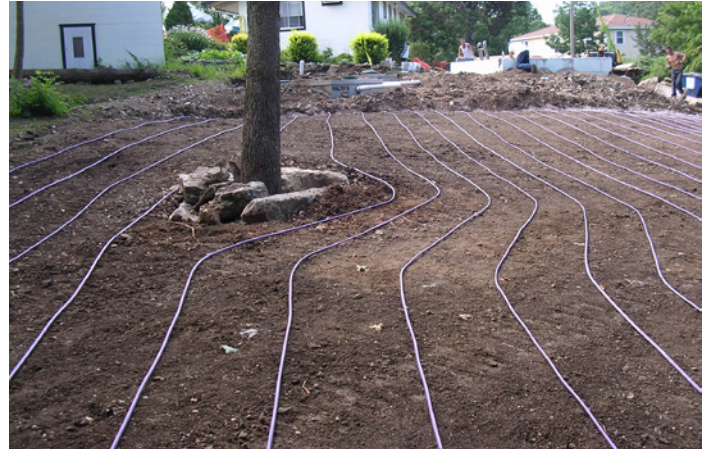
Here is an excellent example of the flexibility of Bioline drip dispersal tubing. It easily allows the designer and installer to adapt to the shape of the dispersal field.
