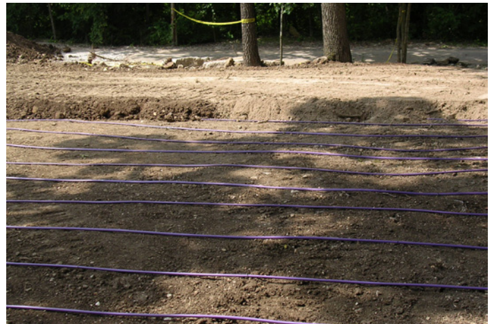
6" soil lifts were used to cover the Bioline in the drip fill. This technique is referred to as 'drip and fill'.
