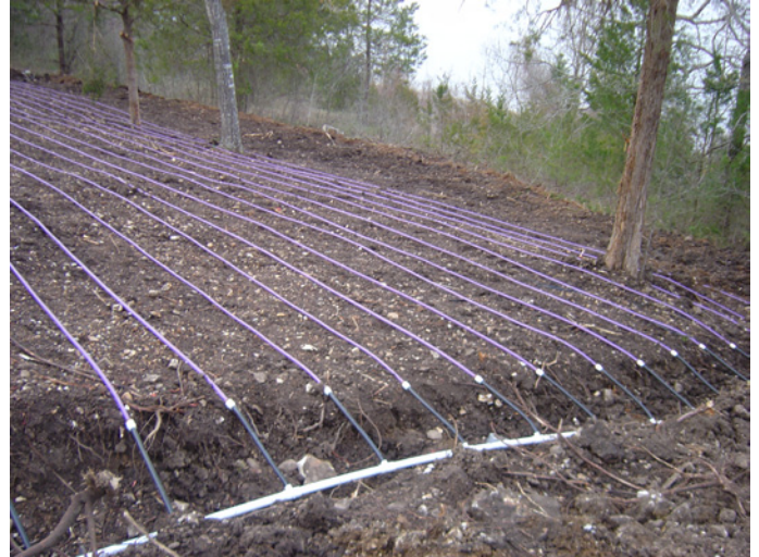
Dripperline is laid in even rows perpendicular to the slope of the field. Note how the tubing passes close to trees that remained in the drip field. Notice the use of flex PVC to transition from the supply and return headers up to the dripperline laterals. This helps to protect the dripperline from damage in poor soils as well as preventing drippers from being placed outside the boundary of the drip field.
