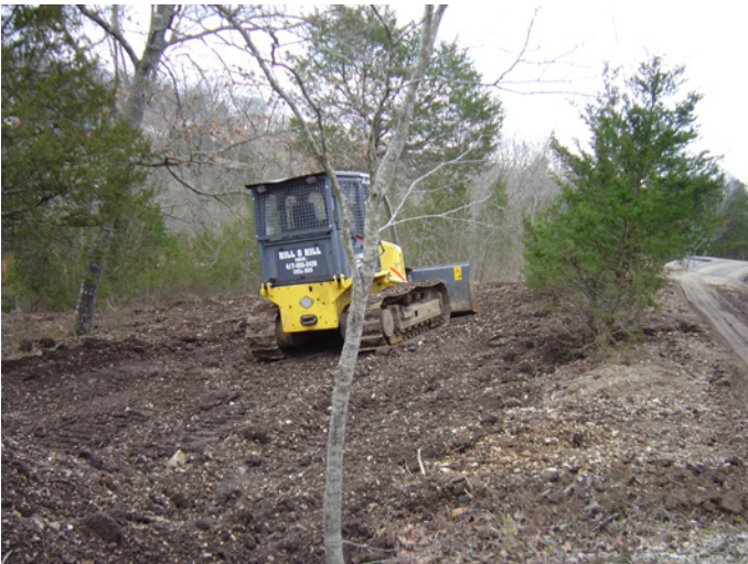
Imported soil is spread across the future drip dispersal field before dripperline is installed. Bringing in soil in 4" to 6" lifts is typical. Total soil depth of approximately 18" was achieved.
