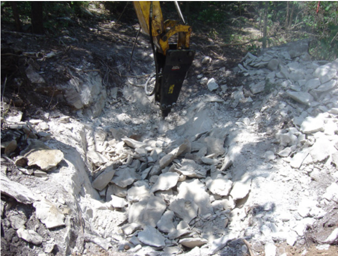
The property did not have a good soil base for the drip field. The drip field required that soil be imported to establish the needed base.
