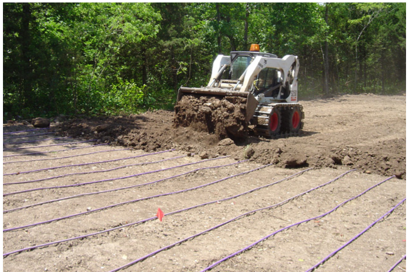
This photo shows the proper method for covering the dripperline in a 'drip and fill' application. The use of a track vehicle to provide a reduced weight footprint is important. As soil is brought onto the field, it is important to keep the vehicle moving with the dripperline to prevent it from shifting.
